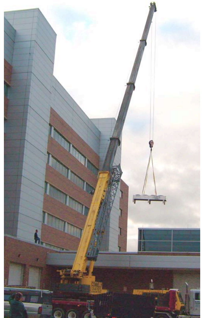
Cooling units being lowered onto the roof above the server room at the BPS building.
